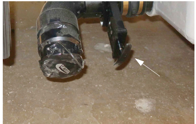
Black Waste Tank Drain Valve (Located in driver side compartment) -Typical View
